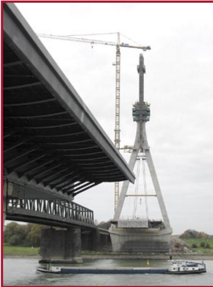
New Rhine Bridge Wesel, Germany. Construction site to be visited by Cruise Boat
