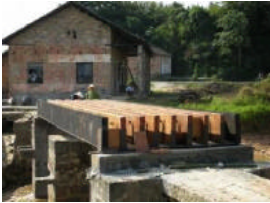
The 10 meter long modern bamboo bridge under construction. (Credit: Yan Xiao, Image courtesy USC Viterbi School of Engineering)
